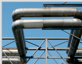
Pipelines subject to pressure
