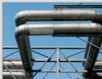
Pipelines subject to pressure
