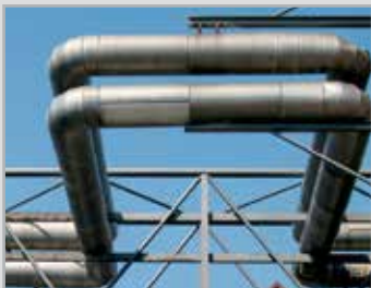
Pipelines subject to pressure
